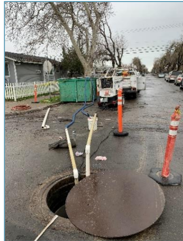
Dewatering 42-inch FRPMP into baker tank for treatment prior to discharge to City sanitary sewer line
