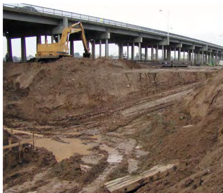
Figure 20. View of the new 9th St Bridge under construction, 2003. The new bridge was being constructed during this study alongside of the old 9th St. bridge, which will eventually be demolished. Bridge work is scheduled to be finished in 2005.
