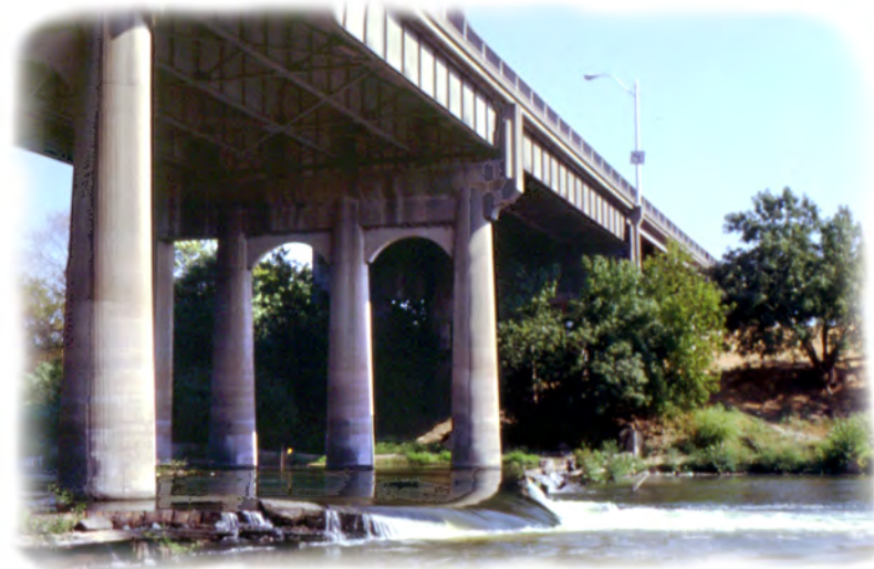
The remnants of Dennett Dam, located under the 9th Street Bridge, currently pose an obstacle to fish migration and impede boat passage. The TRRP Master Plan recommends that it be removed to improve these conditions.
