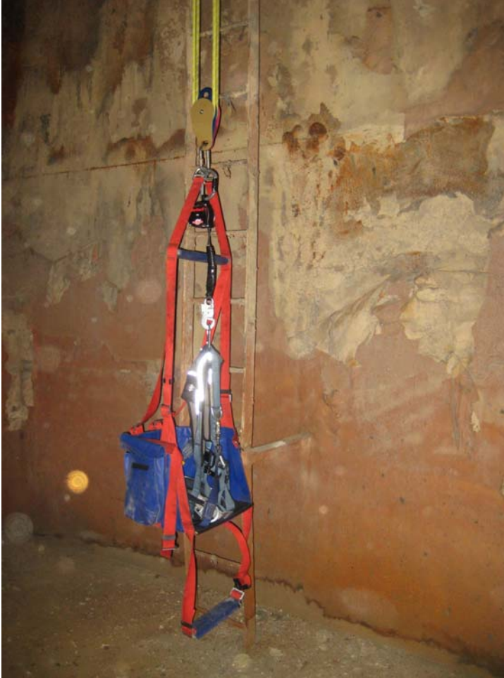
Figure 3-16 Interior of Digester No. 1 (Note: Generally in good condition [note absence of corrosion]).
