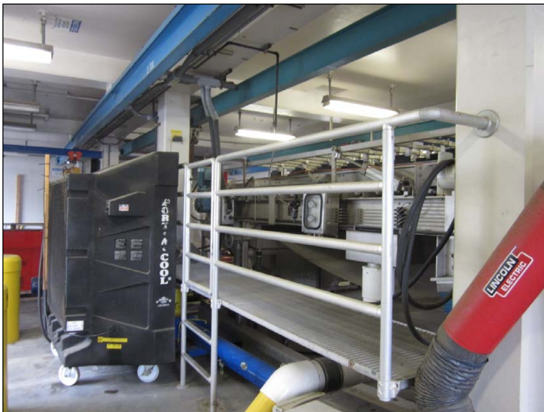
Figure 3-11 Gravity Belt Thickener (GBT) in the DAFT Support Building
