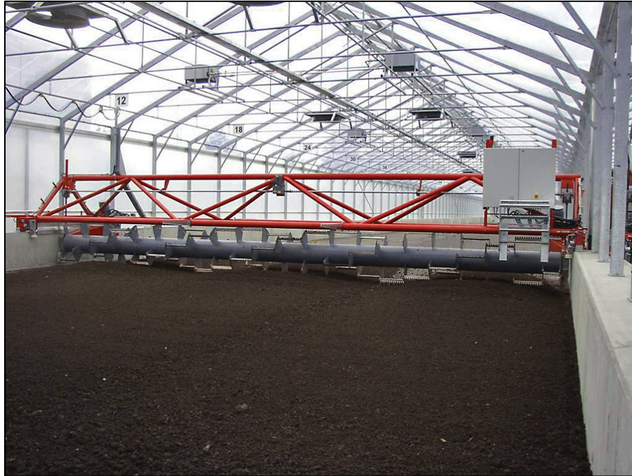
Figure 8-4 Solar Sludge Drying Bed. Image Courtesy of Heliantis™
