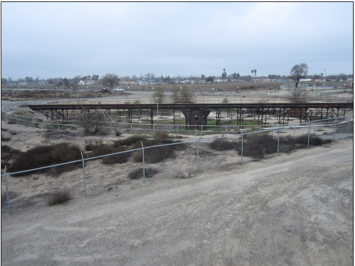
Figure 3-10 Old Abandoned Vortex Aeration Basin
