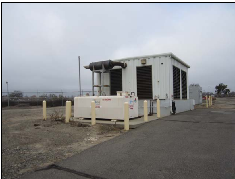
Figure 3-9 Effluent Pump Station Standby Generator
