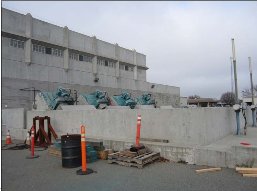
Figure 3-3 Influent screw pumps at Headworks, (looking north).
