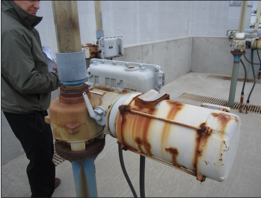
Figure 3-5 Corrosion on a Gate Valve Operator at Headworks
