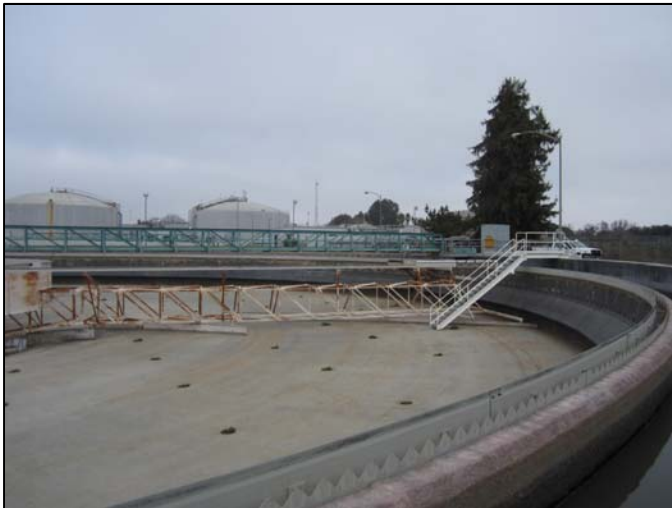
Figure 3-7 Primary Clarifier No. 2 (with Pressure Relief Pipes in the Floor Slab)
