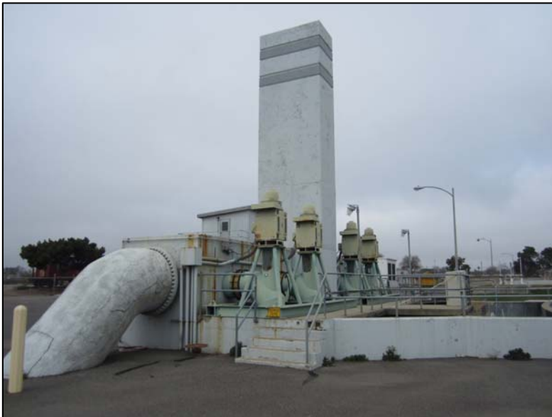
Figure 3-8 Effluent Pump Station with Pump Motors at Higher Elevation
