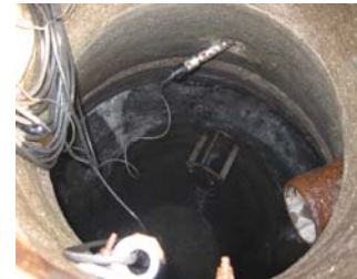
Hahn Lift Station Wetwell
