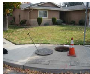
Hahn Lift Station Drywell Access
